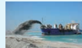
Self-propelling trailing suction hopper dredger, "QUEEN OF PENTA-OCEAN," (currently ANDROMEDA V) put into commission in Singapore (1999)
