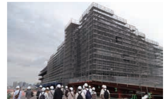
Work site visit held for individual shareholders at new construction of the Tokyo International Cruise Terminal (September 2019)
