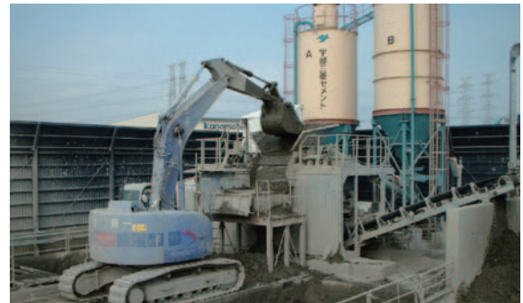
Sludge treatment plant
