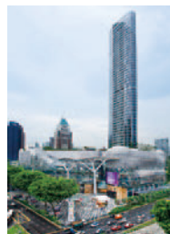
Construction work at the ION Orchard and the Orchard Residences in Singapore
