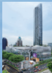
Construction work at the ION Orchard and the Orchard Residences in Singapore
