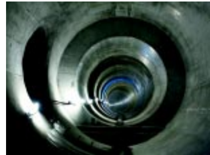
Tamagawa Joryu rainwater main sewerage line
