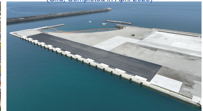
FY2025 Construction Works for Quaywall (-12m) at Karahama District, Sendai Port (Kagoshima, Completed in Mar. 2026)
