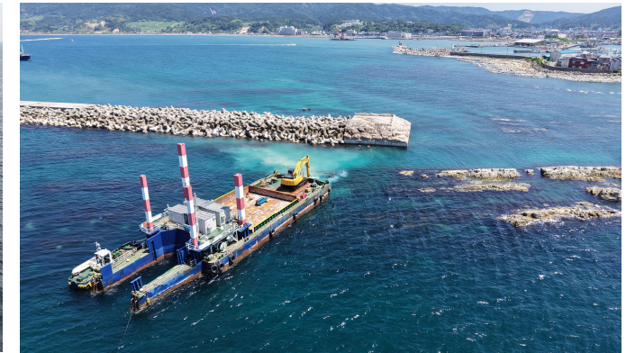
Dredging and One Other Work for Disaster Recovery of Basin (-7.5m) at Kawai District, Wajima Port (Ishikawa, Completed in Mar. 2026)
