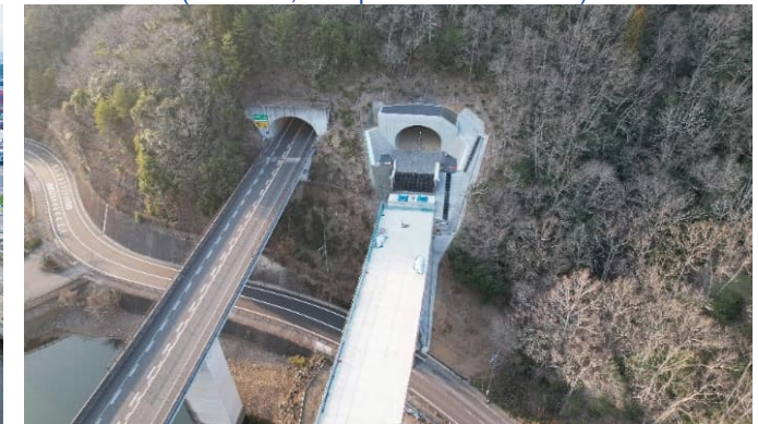
Tokai-Kanjo Expressway Kukuri No.2 Tunnel and One Additional Tunnel Construction Works (Gifu, Completed in April 2025)
