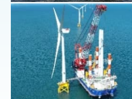
Completion of wind turbine foundations and marine works for the Kitakyushu Hibikinada Offshore Wind Power Project (2025)
