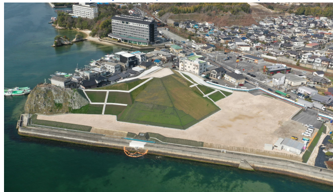
(Tentative Name) Land Development Works for Miyajimaguchi West District (Hiroshima, Completed in Mar. 2026)
