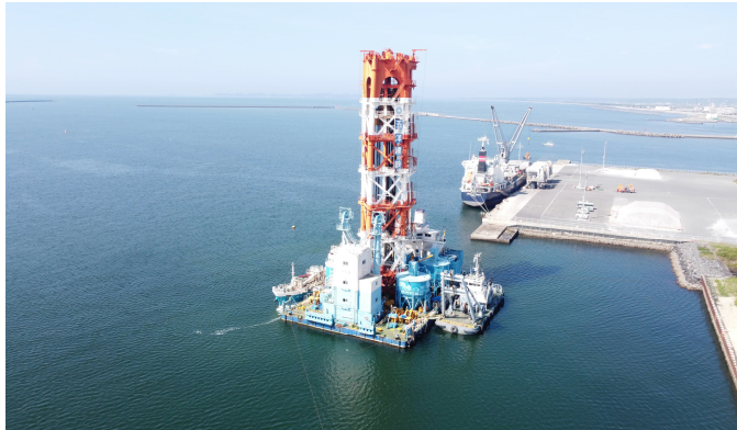
Soil Improvement Works for Earthquake-resistant Quaywall (-12m) at Hibarino District, Ishinomaki Port Area, Sendai-Shiogama Port (Miyagi, Completed in Dec. 2025)
