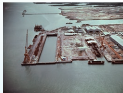
Undertook the construction of the pier at the Jurong Shipyard docks Foray into Singapore (1964)
