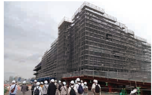
Individual shareholder site visit to the new Tokyo International Cruise Terminal (construction) (September 2019)
