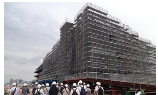
Work site visit held for individual shareholders at new construction of the Tokyo International Cruise Terminal (September 2019)
