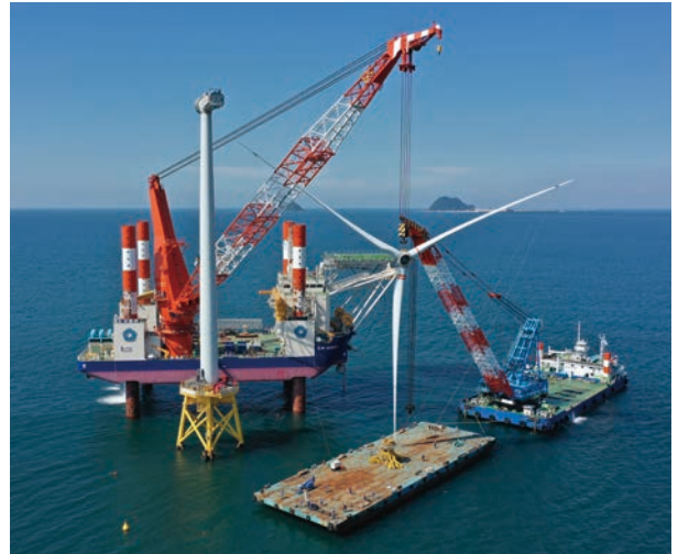
Removal of offshore wind turbines off the coast of Kitakyushu (CP-8001 is the vessel behind the turbines)
