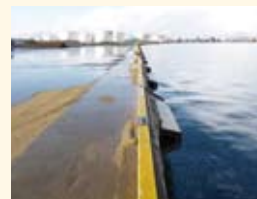
An improved wharf remains in a sound state after the Great East Japan Earthquake
