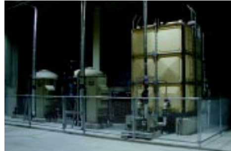
Ultraviolet disinfecting and filtration unit
